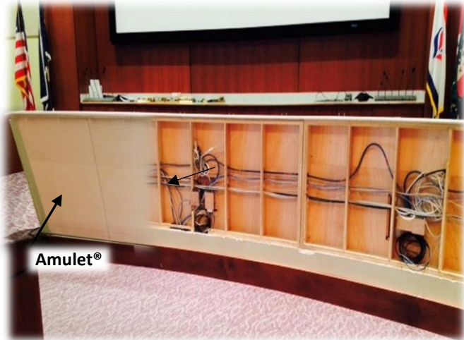
The original Dias wood fascia was removed and Amulet ® Ballistic Barriers was attached to the wood frame (as shown in this photo).
